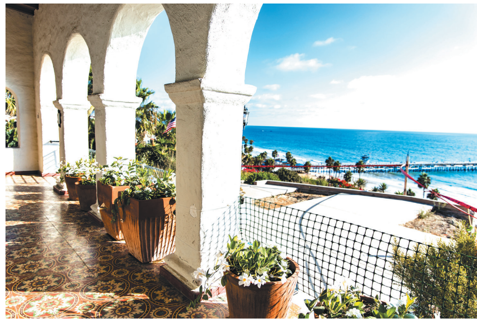
MAIN SALON PATIO: the cement on the other side of the netting fell during the slide.
